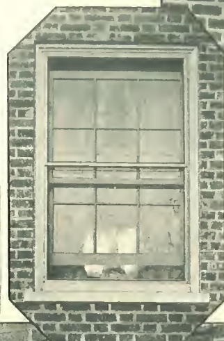
The illustration of double vertical screens (left), shows both top and lower sash partially open, permitting ventilation both top and bottom, but still protected from insects, etc.
